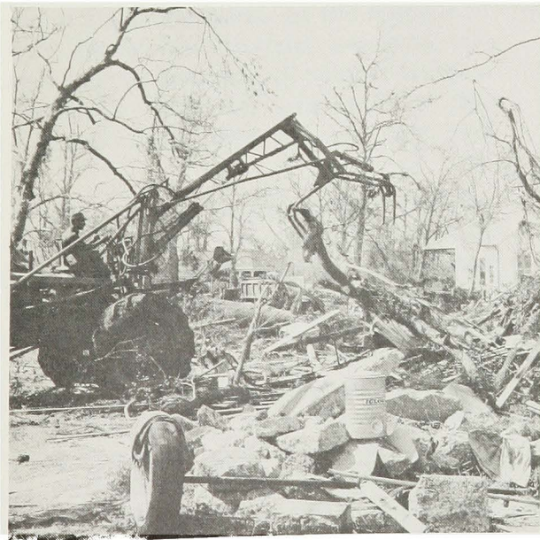
CLEARING PRIVATE PROPERTY OF SAFETY AND HEALTH HAZARDS
