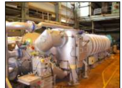
QinetiQ Pyrolysis Waste Destruction System
