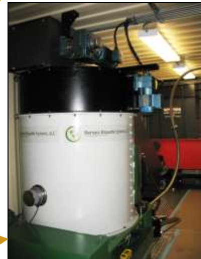
Feedstock Conditioning Module
