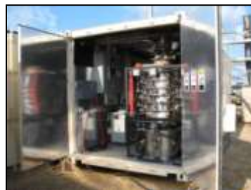
Gas production module (containerized gasifier)
