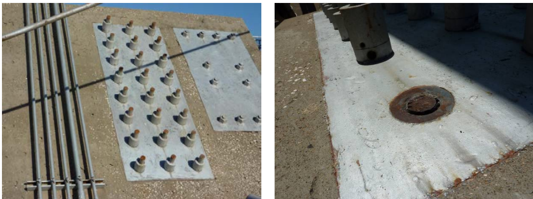
Figure 8. Rod ends at Kaskaskia Lock and Dam (left); broken rod (right).
