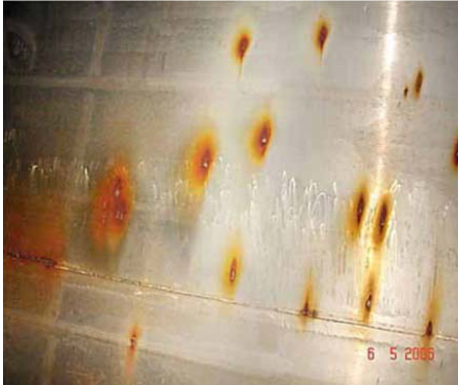
Figure 3. Pitting corrosion observed on a flat wall (Lomas & Callow, 2009).
