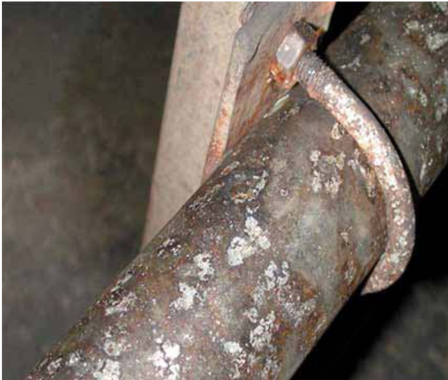
Figure 1. Uniform corrosion observed on a steel piping system exposed to seawater. (Lomas & Callow, 2009)
