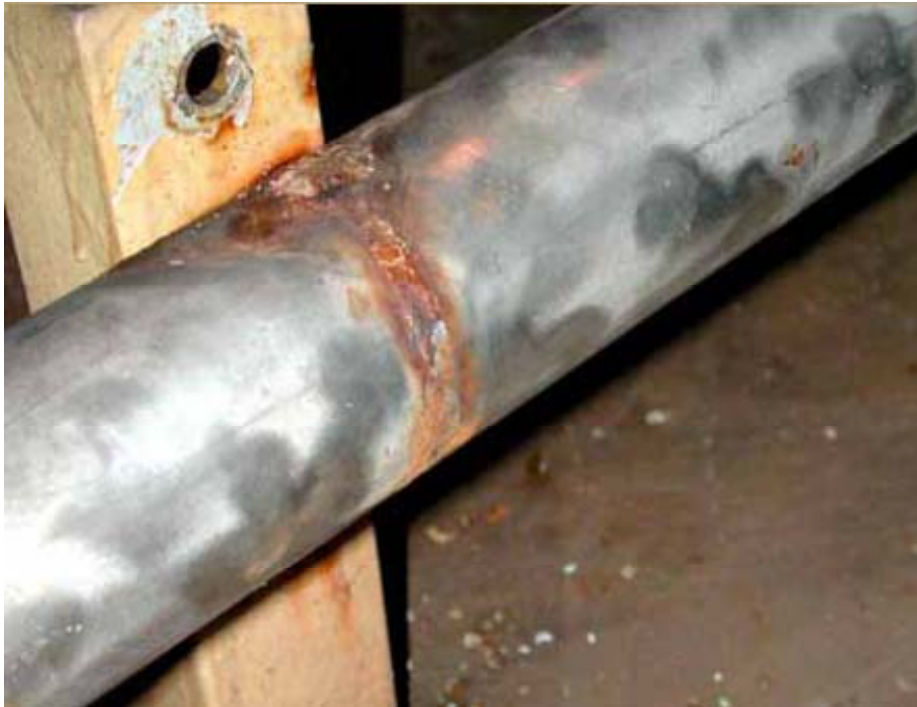
Figure 2. Example of crevice corrosion that developed under a pipe hanger due to stagnant water. (Lomas & Callow, 2009)
