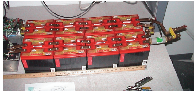
Figure 3. Photo of the 16 PC680 battery bank of the test module.
