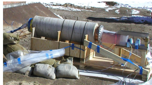
Figure 4. Photograph of Ranchito generator with simulated plate generator load.
