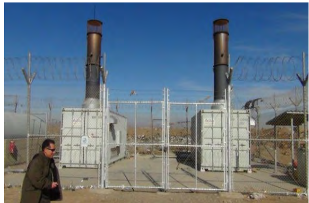
Photo 2 - Afghan-Operated Incinerators Sit Unused Behind a Locked Gate at Shindand Airbase
