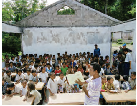
Fatu-Ahi Primary School. Many schools across the country are damaged or unfinished, and lack basic facilities like toilets. Despite this, classes continue.
