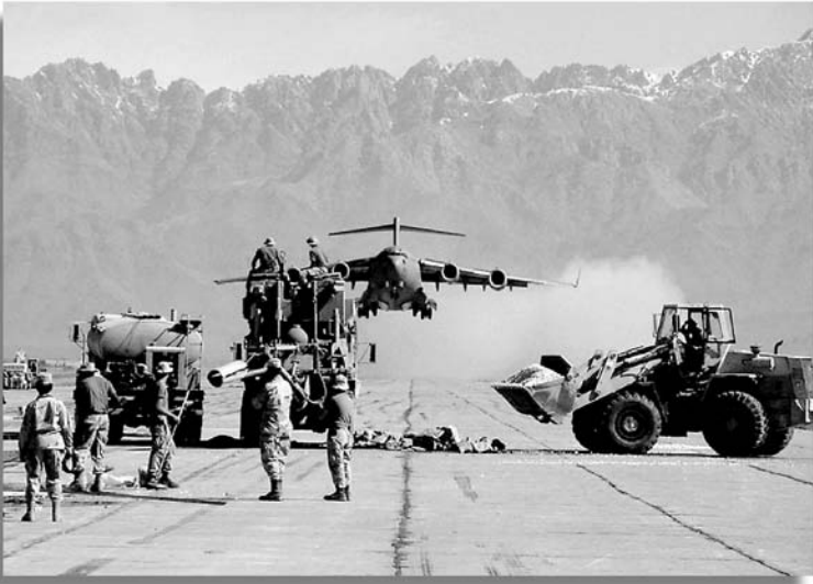
C-17 Globemaster III taking off from Bagram Air Base in Afghanistan while Air Force Civil Engineers repair the end of the runway ( http://www.boeing.com/news/frontiers/archive/2002/may/qt_snapshots.html ).
