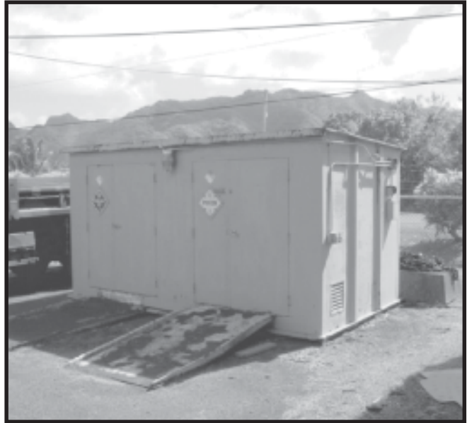
This hazardous materials storage unit should be disposed of. It is unserviceable due to excessive corrosion and weathering.
