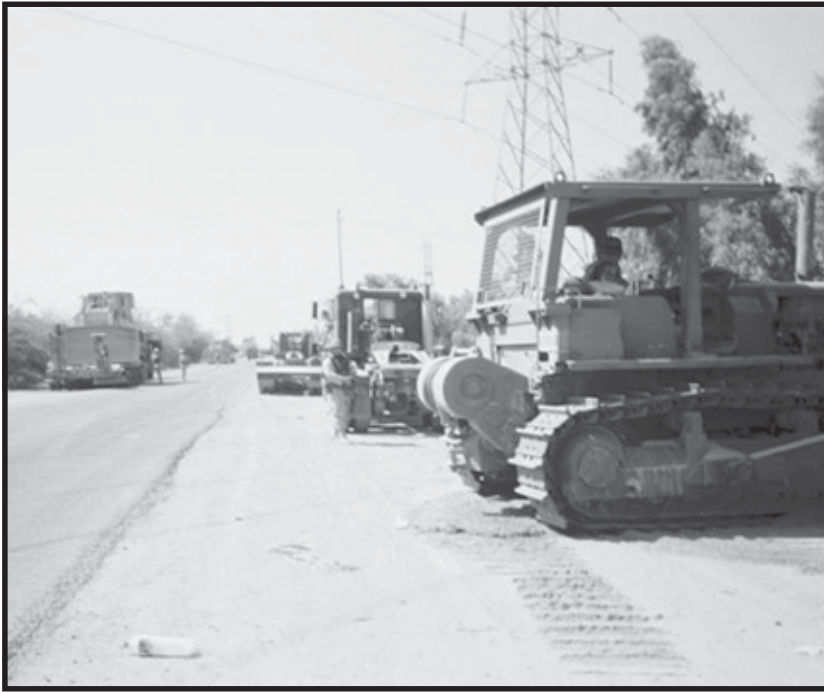
Equipment from the 203d is used to demolish buildings along an alternate supply route.
