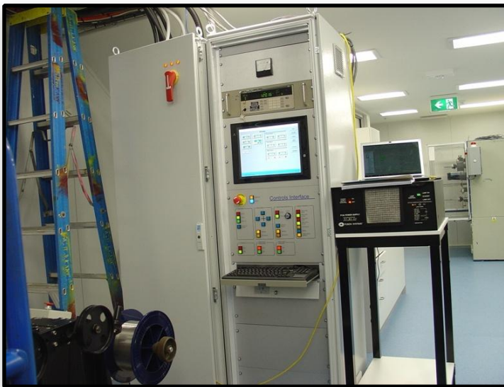
Figure 8: Upgraded all-digital draw tower control unit, which was installed during commissioning.
