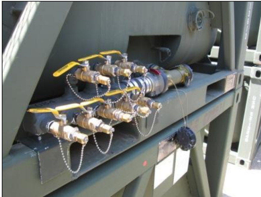
Figure 2-2. Outlet Configuration #1 with Manifold Installed
