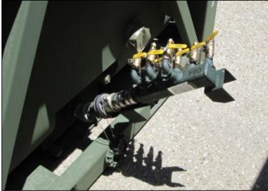
Figure 2-7. Outlet Configuration #3. Manifold Not Properly Oriented or Supported. Manifold Cannot Be Safely Used With This Outlet Configuration
