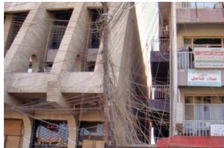
A tangle of consumer-installed electric wires carries power from private generators to households in central Baghdad. (Parsons Brinckerhoff photo)
