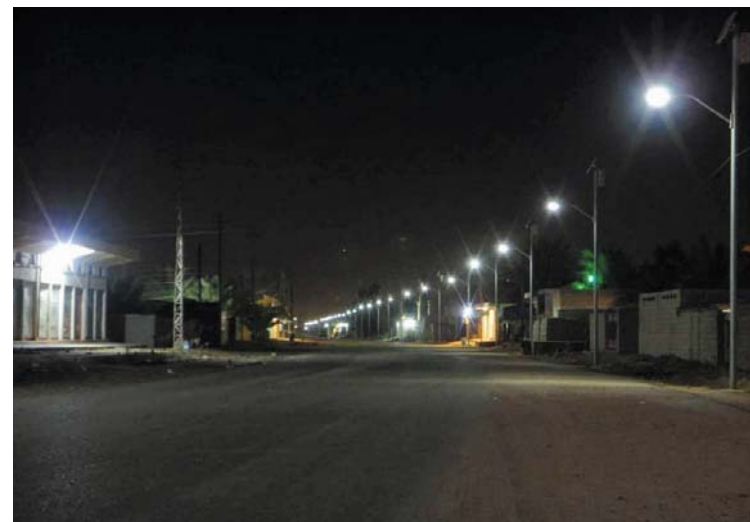
In a $10.2 million, CERP-funded project completed in three phases, USACE installed 1,200 solar-powered street lights along 35 kilometers of roadway in and around Falluja. (USACE photo)
