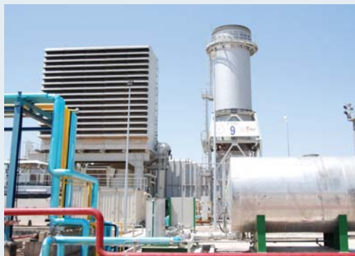
The United States spent more than $250 million restoring the Qudas Power Plant under several different projects. (USACE photo)
