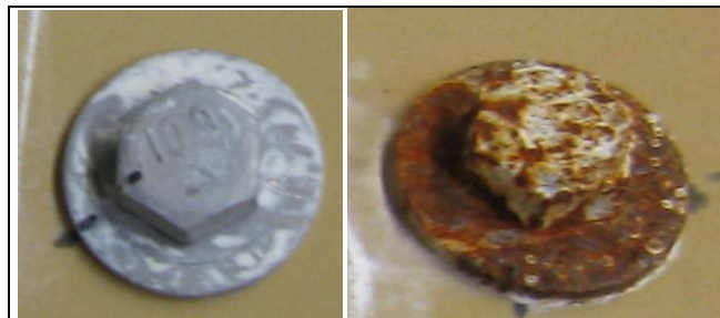
Figure 7. Examples of “frosting” and “red rust.”
