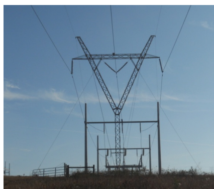
Figure 3. 230 kV Transmission Line
