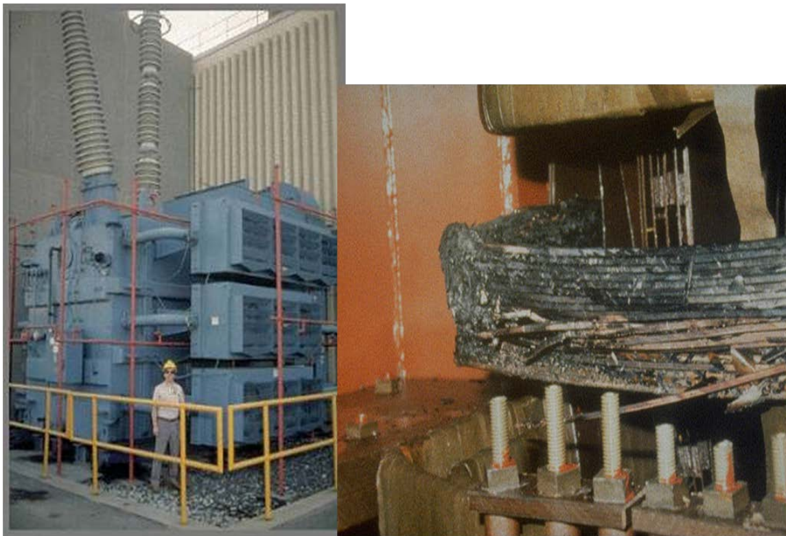
Figure 2. Step-up transformer damaged at Salem Nuclear Generating Plant due to geomagnetic storm on March 13, 1989. Images provided by Public Service Electric and Gas and taken by Peter Balma (pictured). Photograph on the left shows the outside of the damaged transformer for scale. Photograph on the right shows some of the physical damage to the internal components of the transformer.
