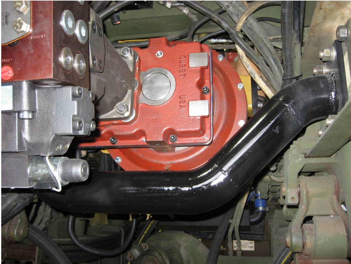
Figure 3.4.1-3. Engine Driven Pump and New Cross-member
