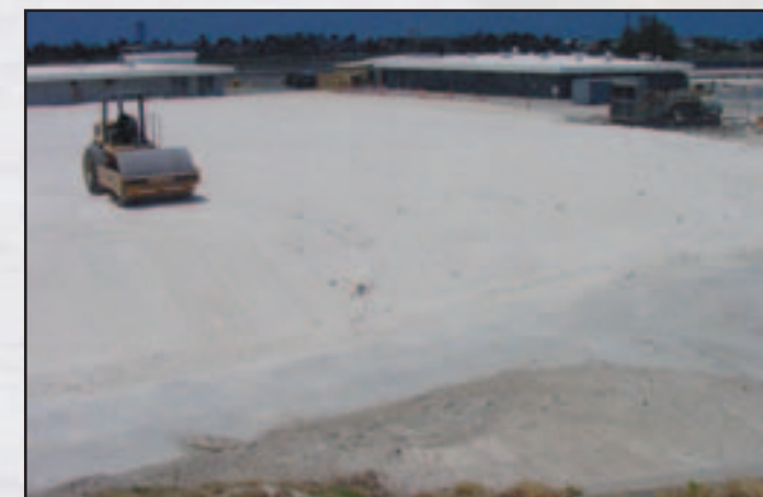
Creating a coral cap over the former site of the Munitions Demilitarization Building (MDB).
