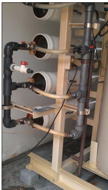
Figure 3. Reverse osmosis water purification system in a bottled water plant.
