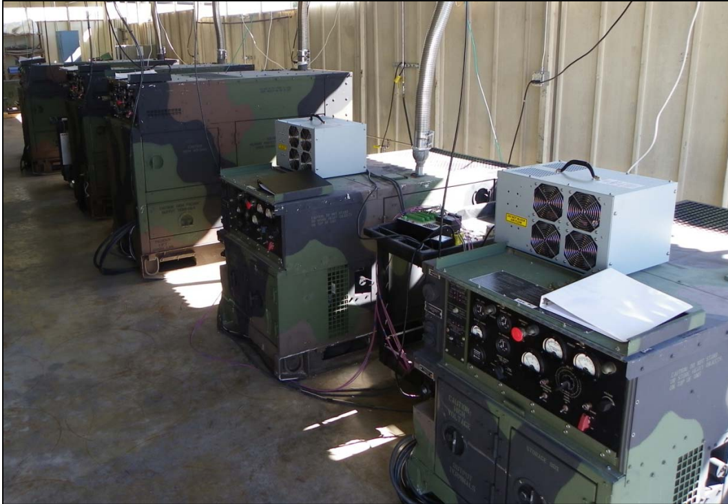
Figure 1. 10kW and 30kW Generators Ready for Testing
