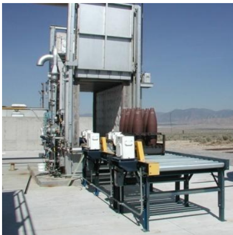
Artillery projectiles being fed into Metal Parts Flashing Furnace
