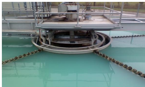
Section of current Lake City AAP Wastewater Treatment Plant
