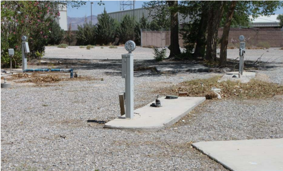
Photo 17. Utilities infrastructure in trailer/RV park.
