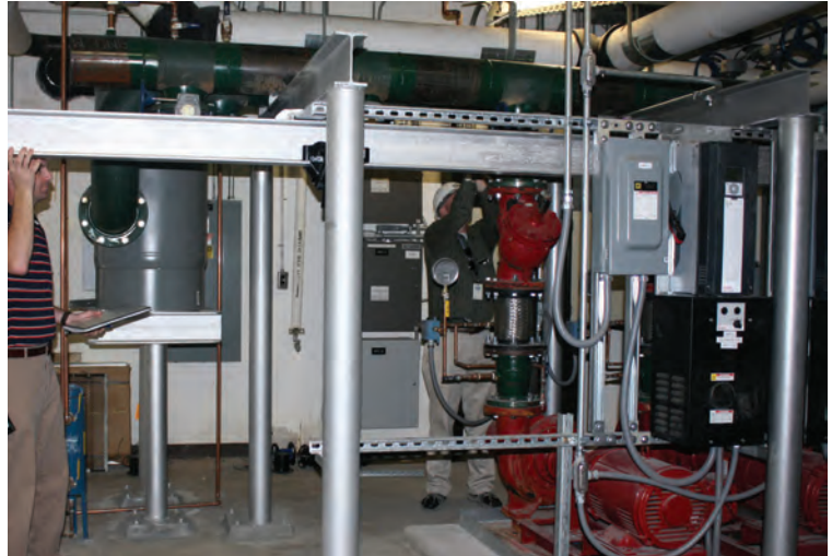
Facilities personnel oversee implementation of Center's secondary "cold" chilled water loop that will increase efficiency and flexibility
