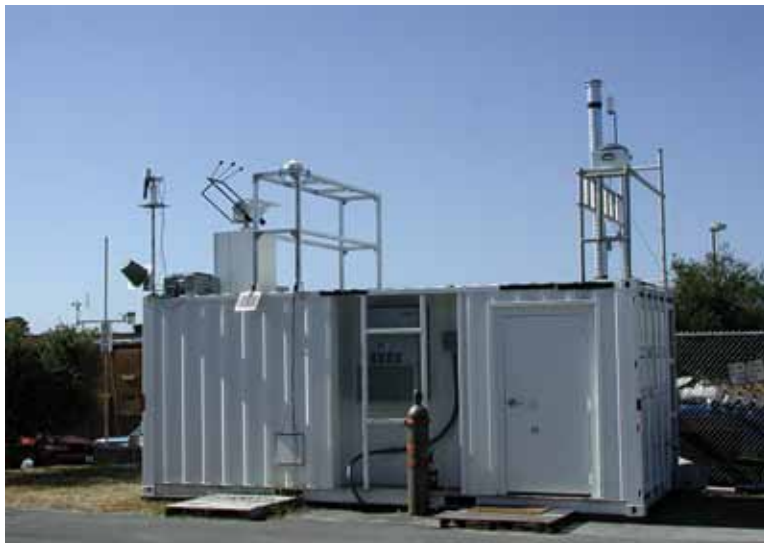
MAARCO is designed as a stand-alone facility for basic atmospheric research and the collection of data to assist in validating aerosol and weather models. Its purpose is to enable research on atmospheric aerosols, gases, and radiation (visible and IR light) in areas of key interest, including remote areas, overseas locales, and onboard ships. This complete mobile laboratory facilitates deployment in areas with limited facilities, and provides maximum flexibility for integration of additional instrumentation.
