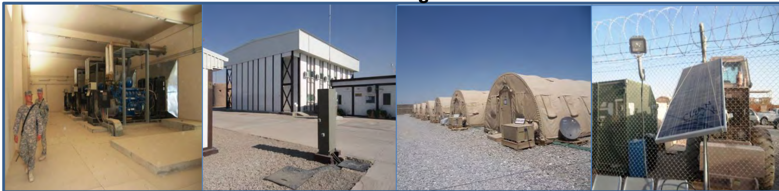
KAF 3MW Plant
