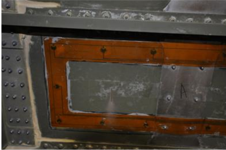
Figure 37. Close up View of Sensors
