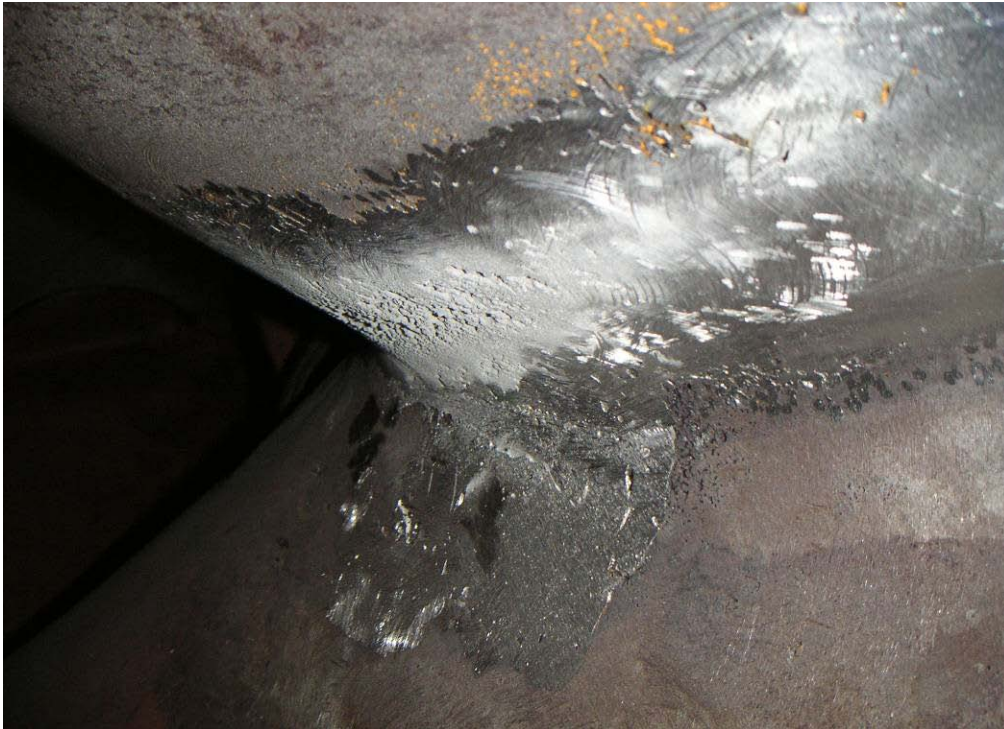
Figure 2. Typical cavitation damage areas on upper one-third of suction side of buckets after approximately 1 year of operation since last repair.
