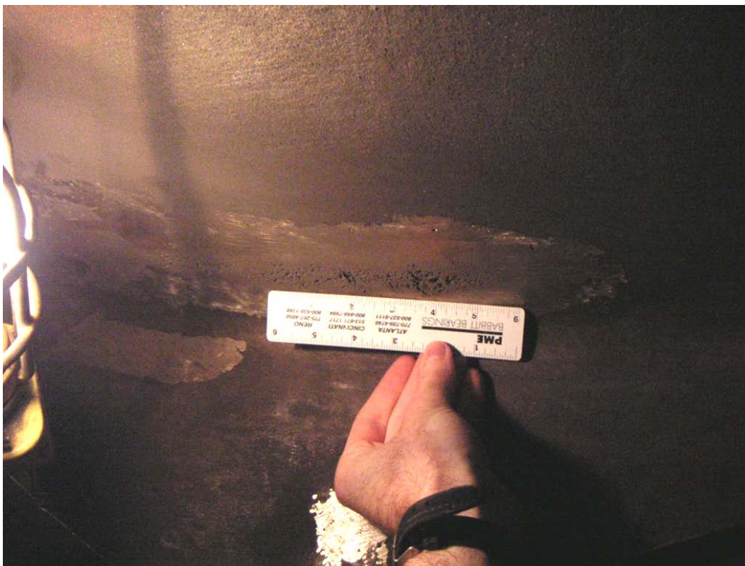
Figure 1. Typical cavitation damage areas on lower one-third of suction side of buckets after approximately 1 year of operation since last repair.
