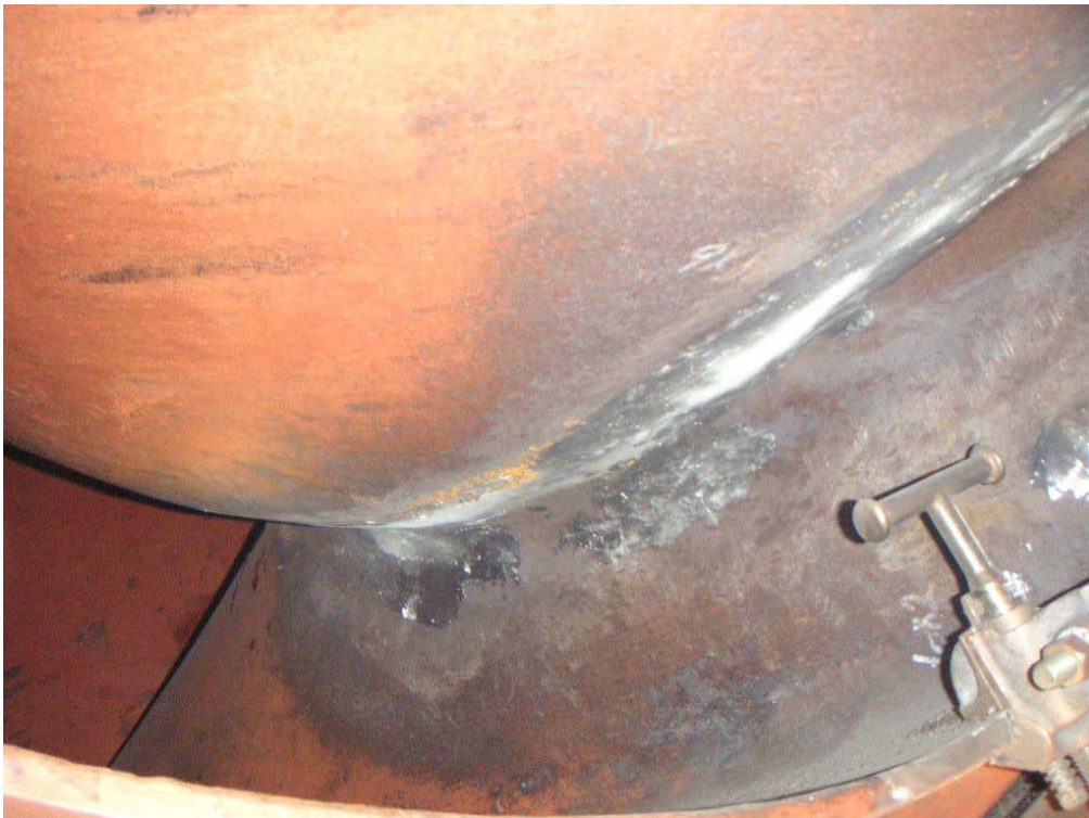
Figure 3. Typical cavitation damage area showing that cavitation-prone area covers much of area near fillet on suction side of buckets.
