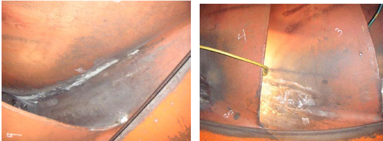
Figure 4. Typical cavitation repair areas on discharge side of buckets.
