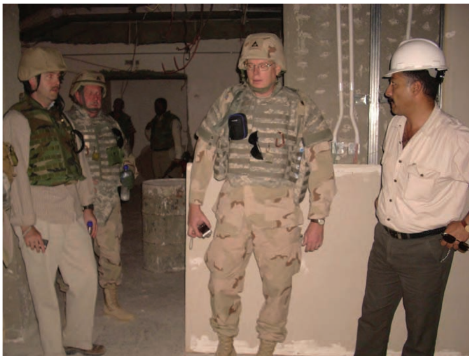
Iraqi construction supervisor guides U.S. contractors through hospital under construction in Basra
