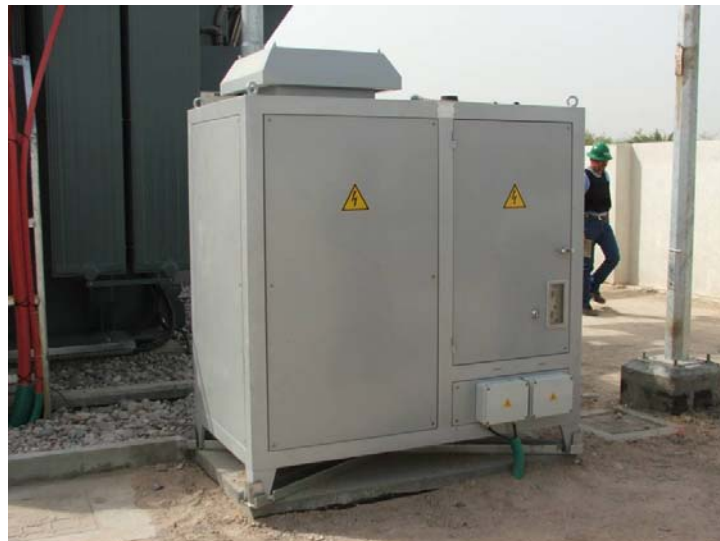
Site Photo 7: Grounding system
