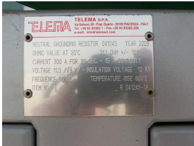
Site Photo 8: Factory nameplate of grounding system
