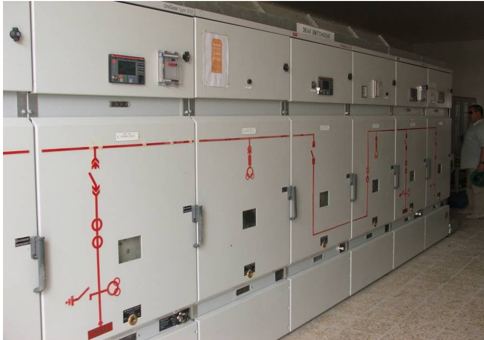
Site Photo 1: 33 kV Switchgear
