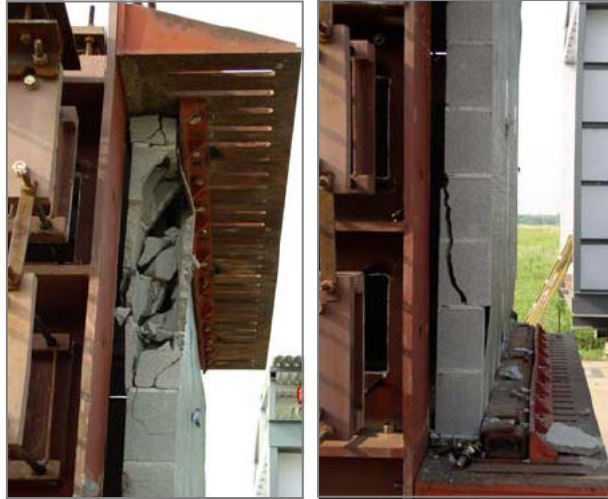
Figure 4. Shear damage to CMU walls upgraded with FRP (BakerRisk, 2003)
