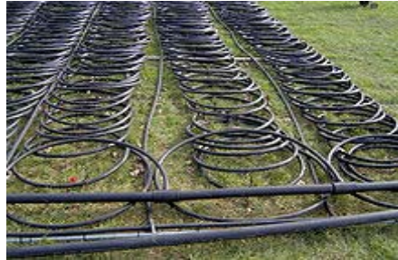
Tubing for Horizontal GSHP
