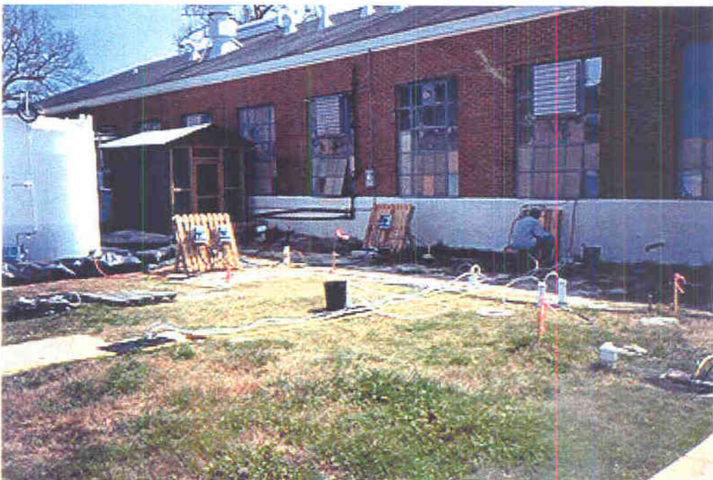
View of the SEAR Demonstration Wellfield facing southeast Left - black mat is on HC01, the pallet parallel to the shed is behind EX06; Center- Black bucket is on IN03, the flagged stake behind this is EX05, and the white disc to the right of the bucket is MW10IW, the pallet against the building is next to EX04R; Right - the pallet with the person in front is next to IN01, the black mat at the bottom right is on EX03
