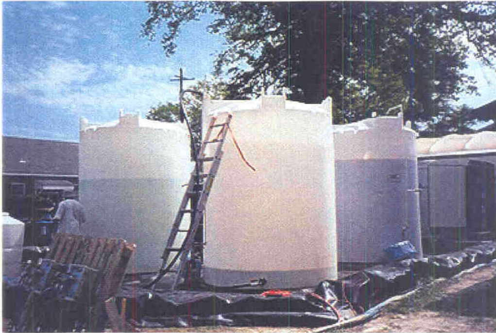
The surfactant tank farm showing on the right the first recycled surfactant tank batch (Tank A) prepared for reinjection
