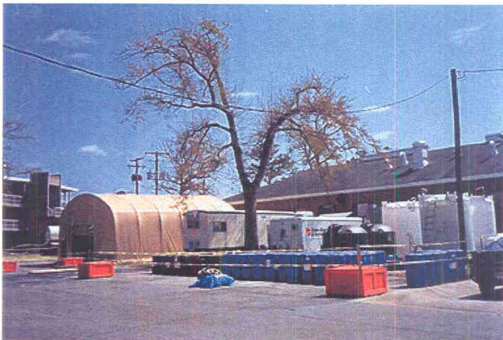
Overall site photo showing from left to right: the surfactant recovery processes tent, the analytical/office trailer, the control trailer and the tank farm
