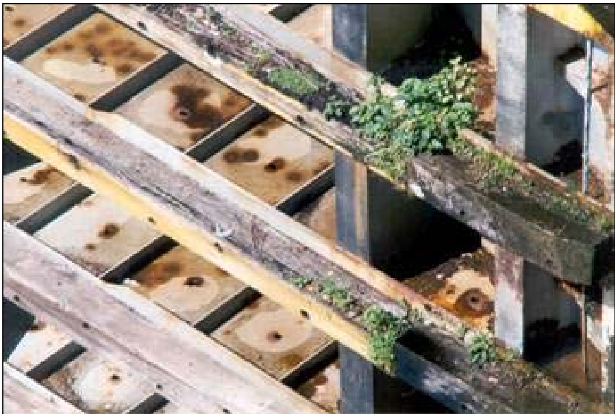
Figure 1. Corrosion on miter gate.
