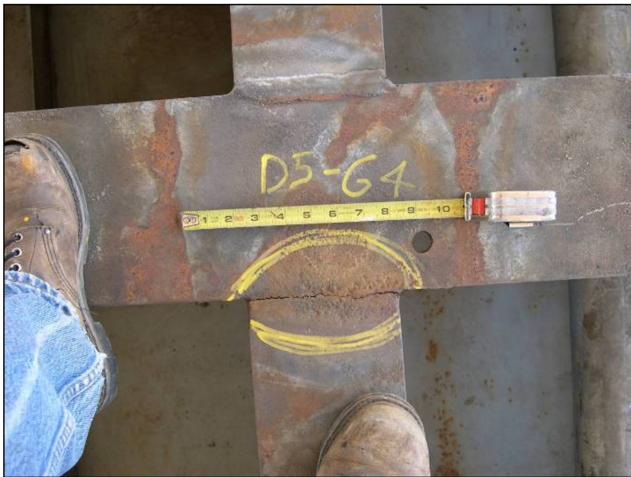
Figure 6. Fatigue crack in diaphragm flanges of miter gate.
