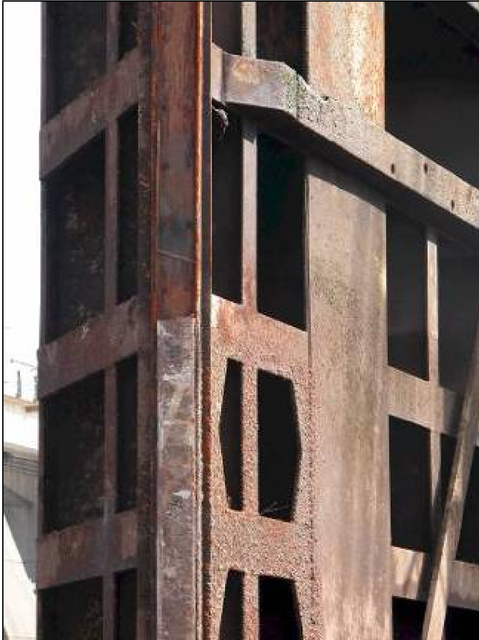
Figure 3. Quoin block failure.
