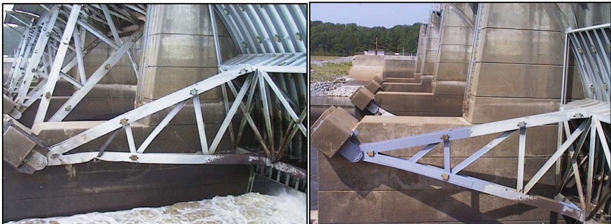
Figure 5. Tainter gate with strut arm damage from barge impact before (left) and after (right) repairs.
