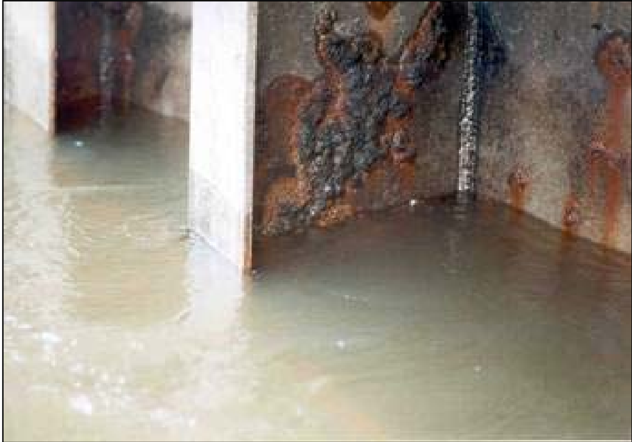
Figure 2. Corrosion inside a lock miter gate compartment.
