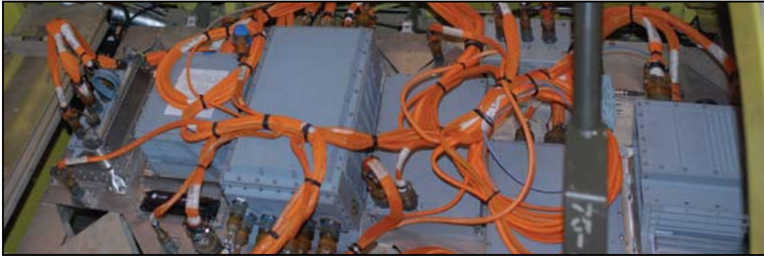
FIGURE 1 CHLOE processing equipment mounted in upper ER-2 Q-bay.
