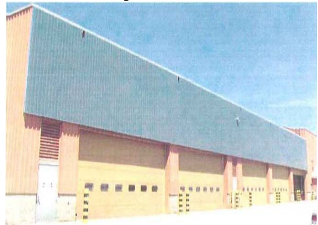
Figure 2. Solar Walls Installed on a Maintenance Shop at Fort Drum
