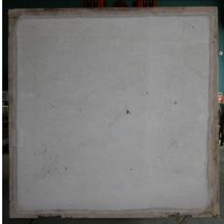
Figure 5. Photograph of the heated face of a 4'×4'×6" geopolymer concrete sample (cured for 7 days after pouring) following exposure to the Standard Time-Temperature Curve heating profile for 4 hours. Note the absence of spalling; this is typical of all samples tested.
