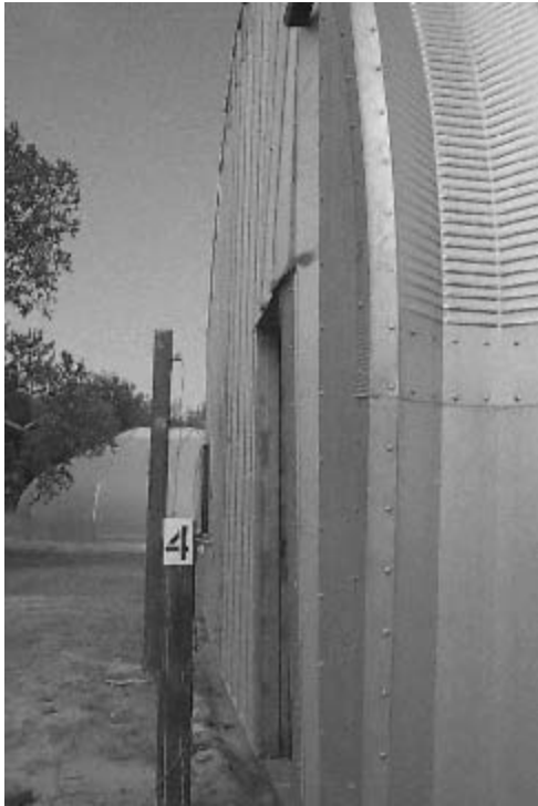
Figure 3 - Personnel Door Damage
