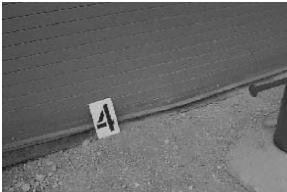
Figure 4 - Roll-up Door Damage
