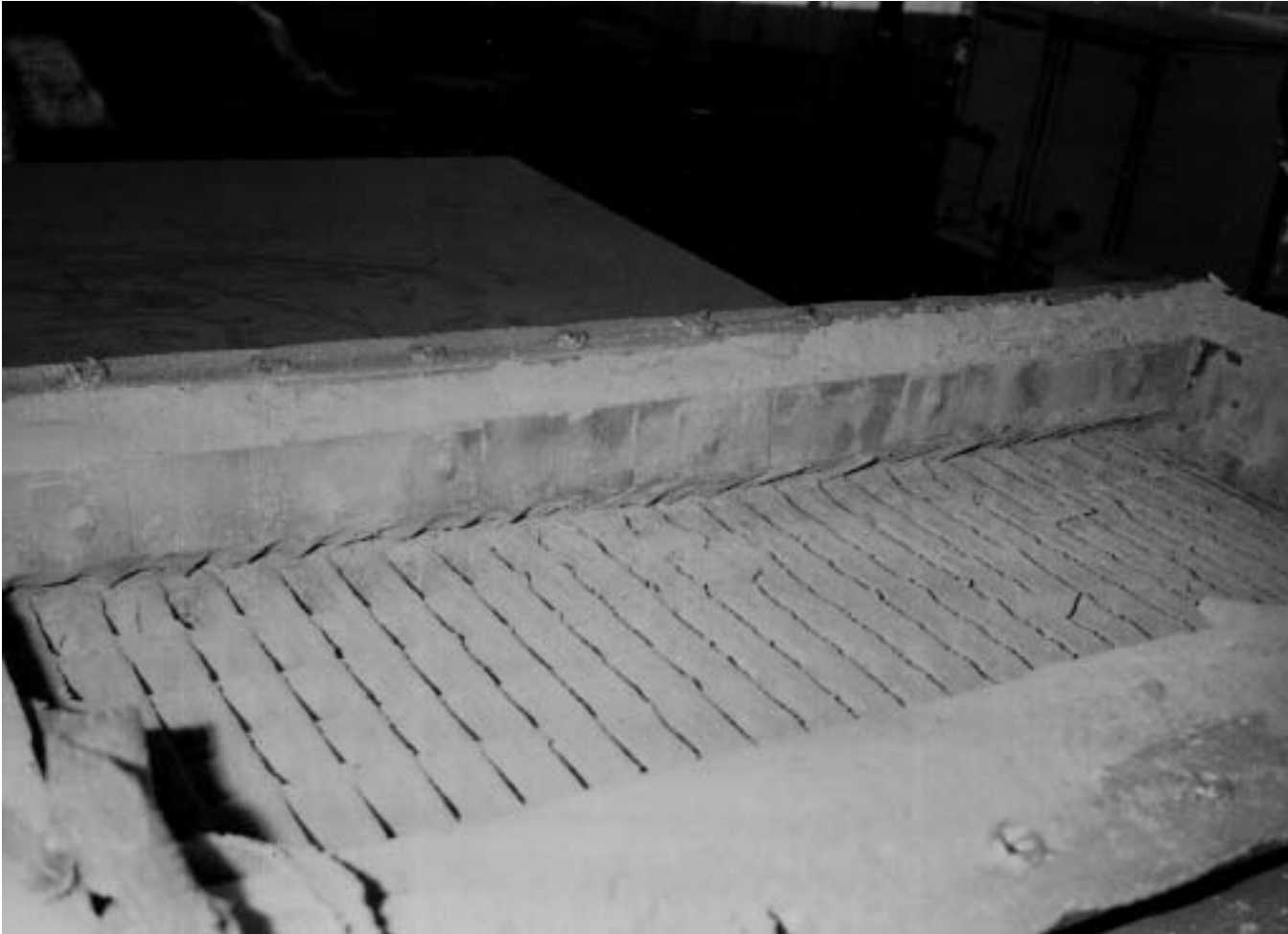
FIGURE 3: TOP VIEW OF CLOGGED HIGH TEMPERATURE GAS COOLER
