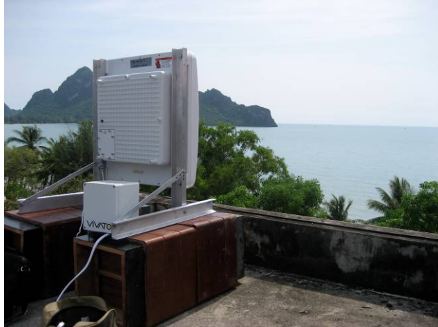
Figure 44. Wireless base station overlooking south bay, from the 4th floor roof access of the Ao Manao Hotel.
