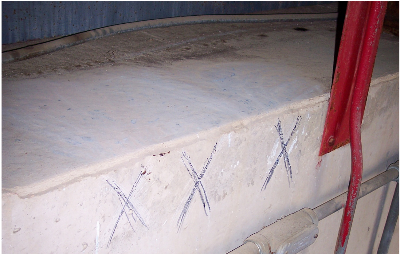
Figure 7-15. Photograph of Contaminated Concrete Ledge Area in Shelter 210.
