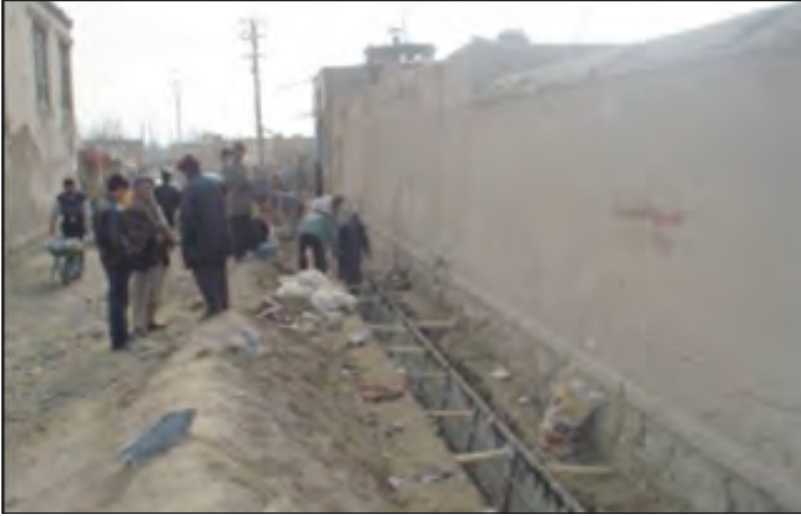
Figure 41. Drainage is a Key Community Improvement. Source: LTERA.
