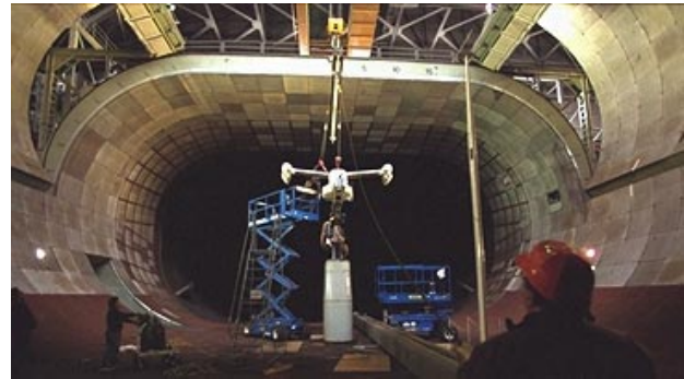
Figure 10. The TRAM is lifted into the 40-by 80-Foot Wind Tunnel Test Section. Clamshell doors are shown partially open.
