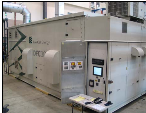
Figure 2. DFC300A fuel cell power plant operating on propane at CTC.
