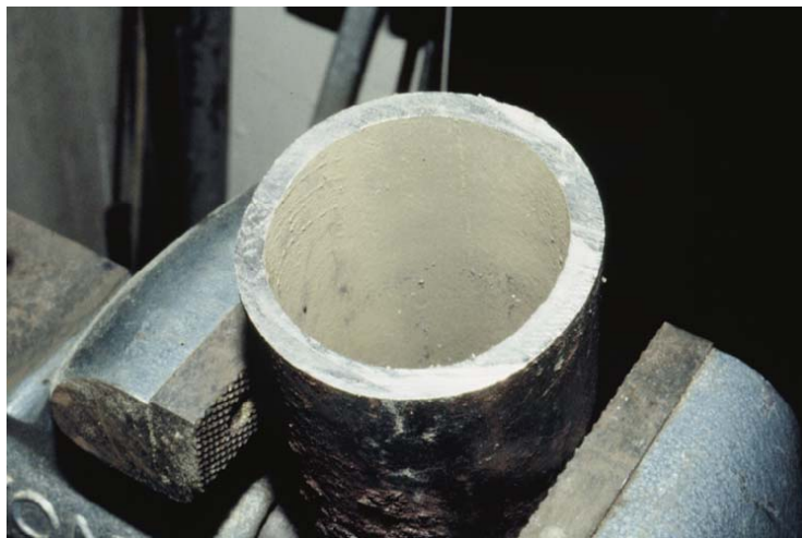
Figure 4. System piping treated with nitrite/borate/azole.
