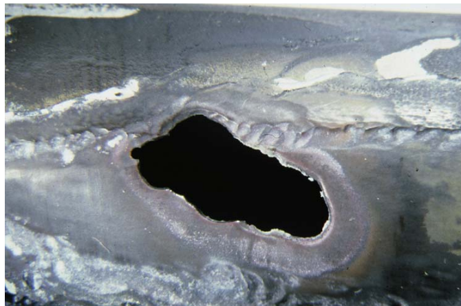
Figure 3. Hot water boiler tube pitting.
