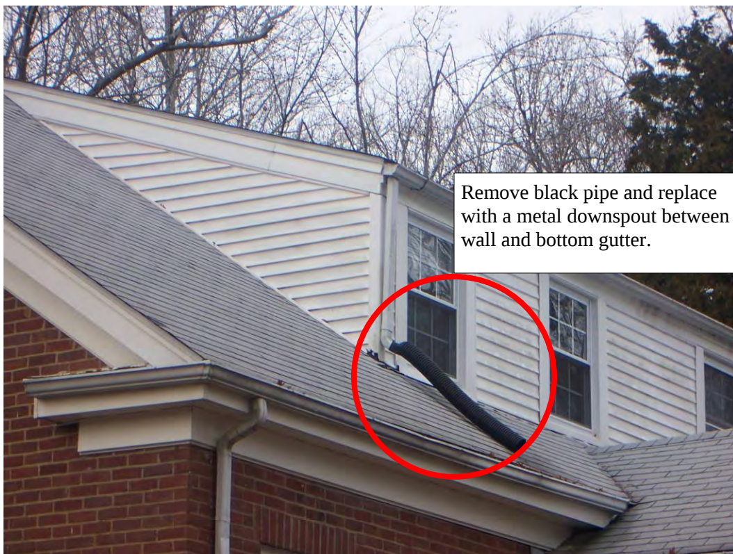
Figure 134. Plastic pipe that ends before gutter.
