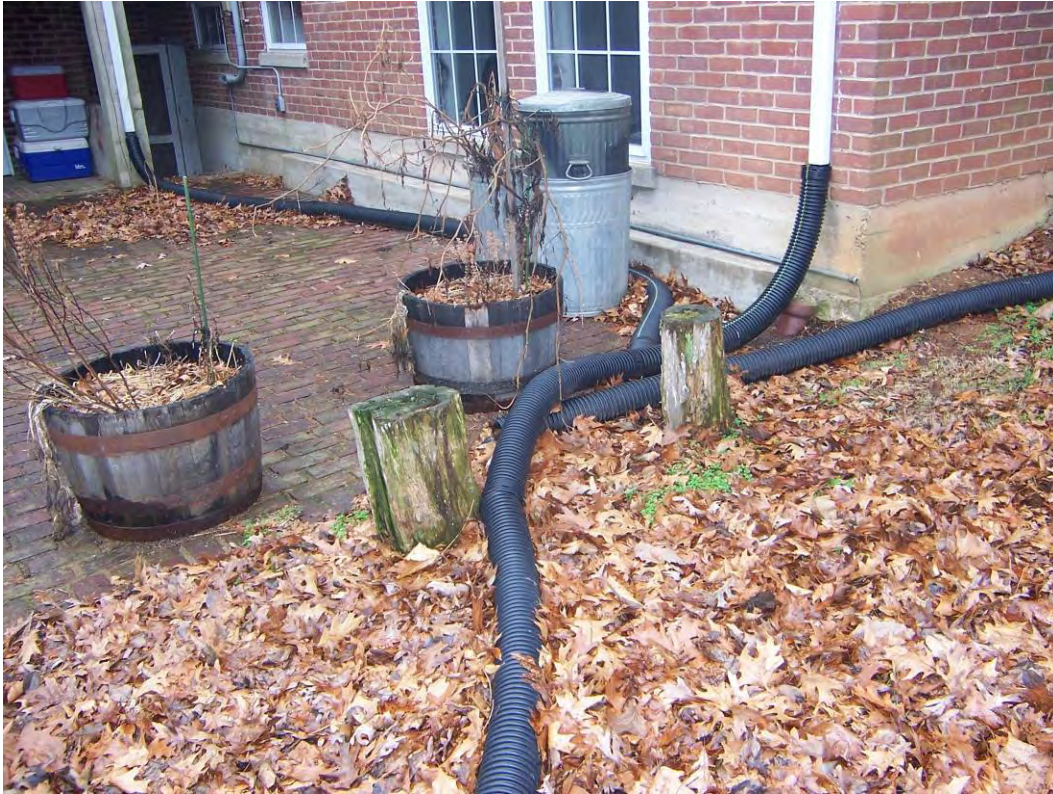
Figure 133. Plastic pipes snaking across patio.
