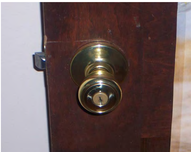
Figure 169. Replacement doorknob in first floor bedroom.
