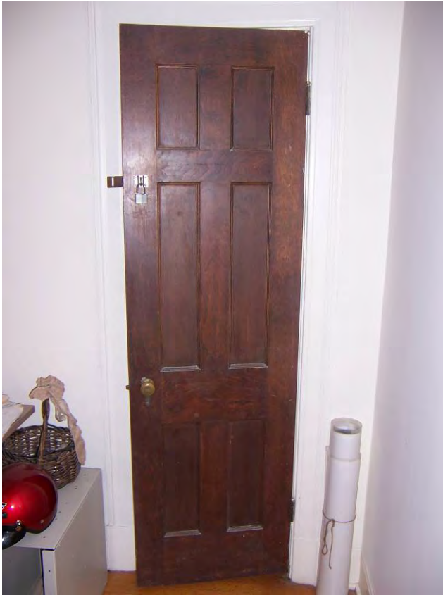
Figure 92. Stained closet door in northeast bedroom.
