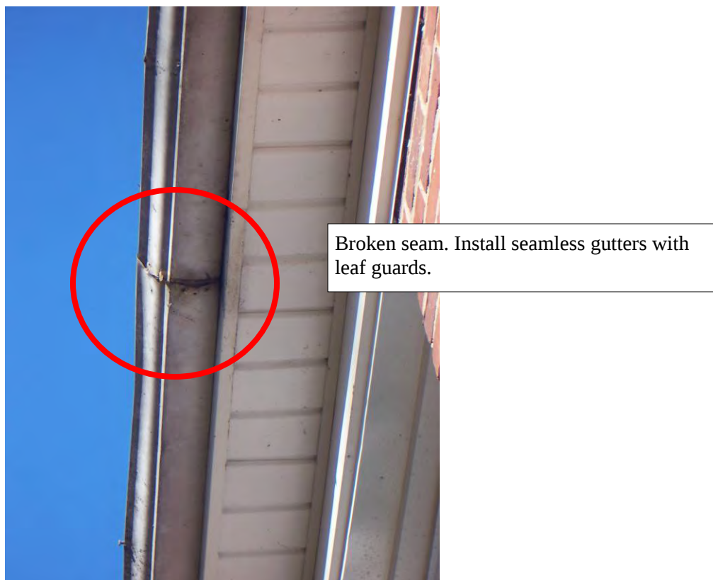
Figure 142. Gutter seal broken between two sections.
