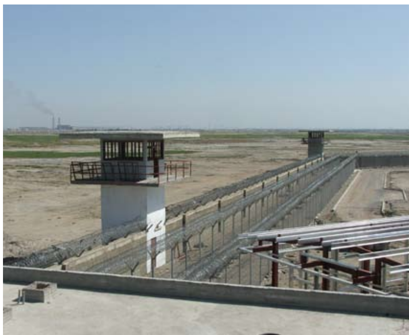
Prison perimeter wall, interior fencing, and guard towers at the Nasiriyah Prison
