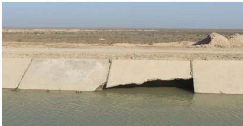
Example of under-cutting of canal
