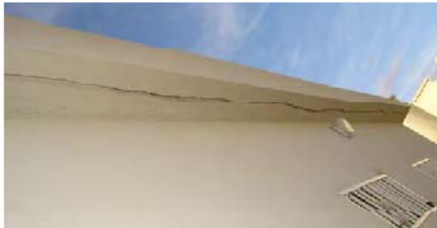
Crack in overhang of border post
