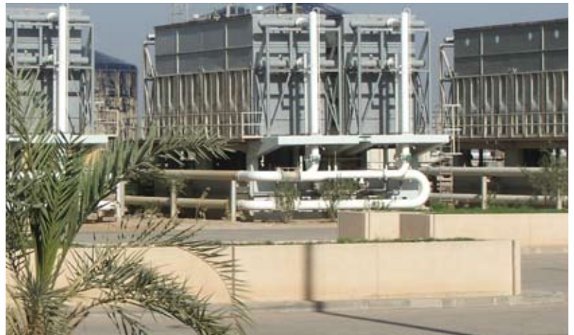
Three pairs of cooling towers for HVAC system of main passenger terminal
