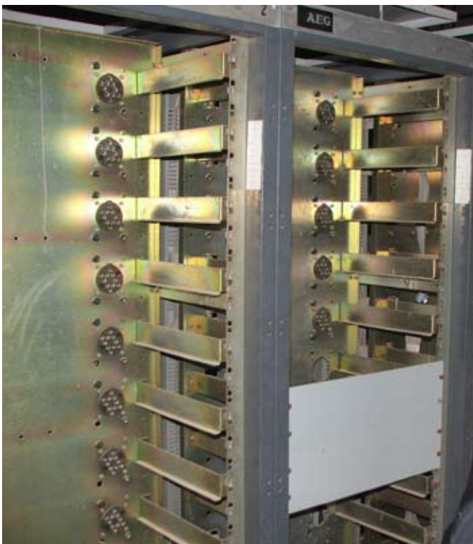
Missing electronic equipment at runway substation
