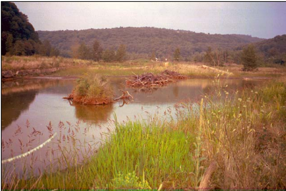
Figure 18. Treated water leaves wetland Area 3b and enters Area 4. The substrate blend consists of bony, waste paper fiber, mushroom compost and Bionsoil™.
