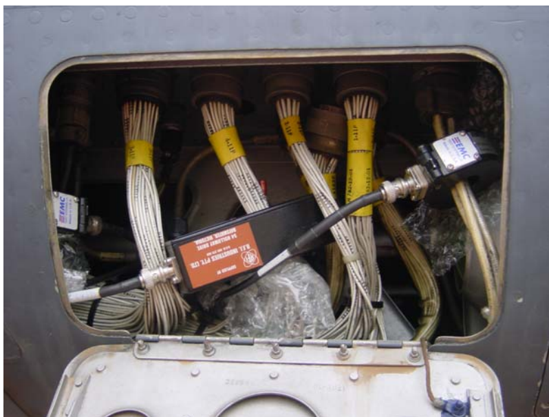
Figure 65 Current clamp locations for inputs 5, 6, and 7. It is behind access hatch AC54, on the starboard side beneath the cockpit.
