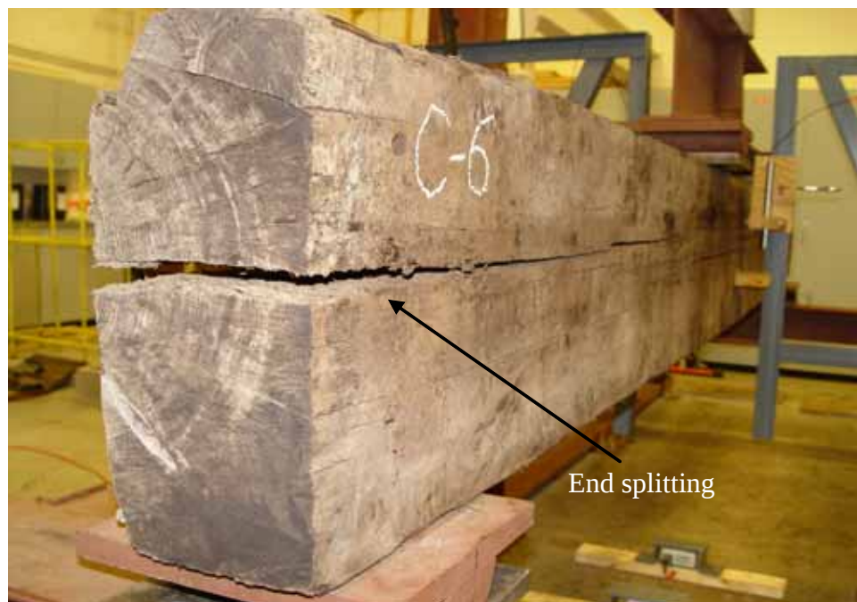
Figure 10. Timber stringers with end splits.
