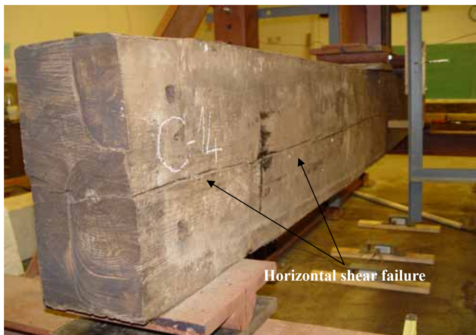
Figure 91. Horizontal shear failure on stringer C14.
